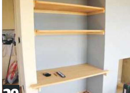
20 Place all shelves on supports. Secure with screws through rear edges down into support battens
